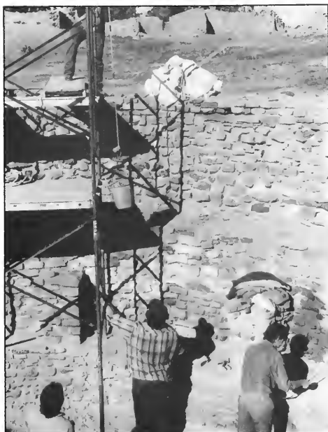
Figure 12.8. Routine maintenance stabilization at Aztec Ruins being done in connection with regional training exercises, May 1989.
